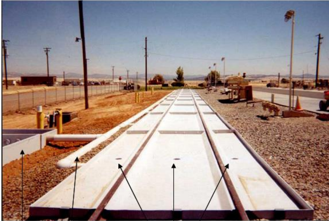
RESERVIOR COLLECTION PIPE 6" MANIFOLD
